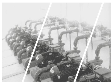
Boosting and Distribution of surface water
