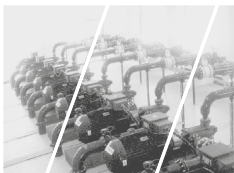
Boosting and Distribution of surface water
